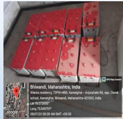
BATTERY BACK -UP
