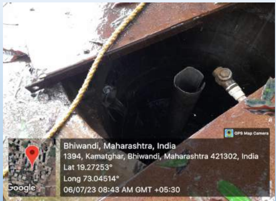
RAIN WATER STORAGE TANK (BOREWELL IN GROUND)
